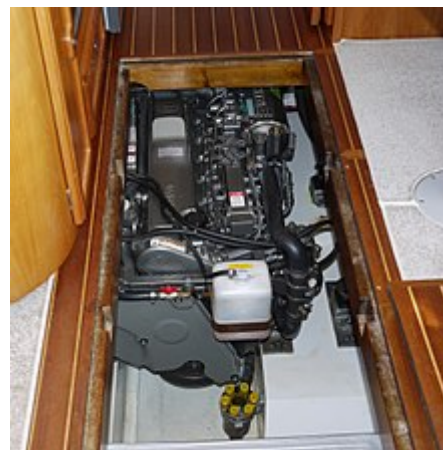
Yanmar 6LPA engine installation in a Corvette 320
